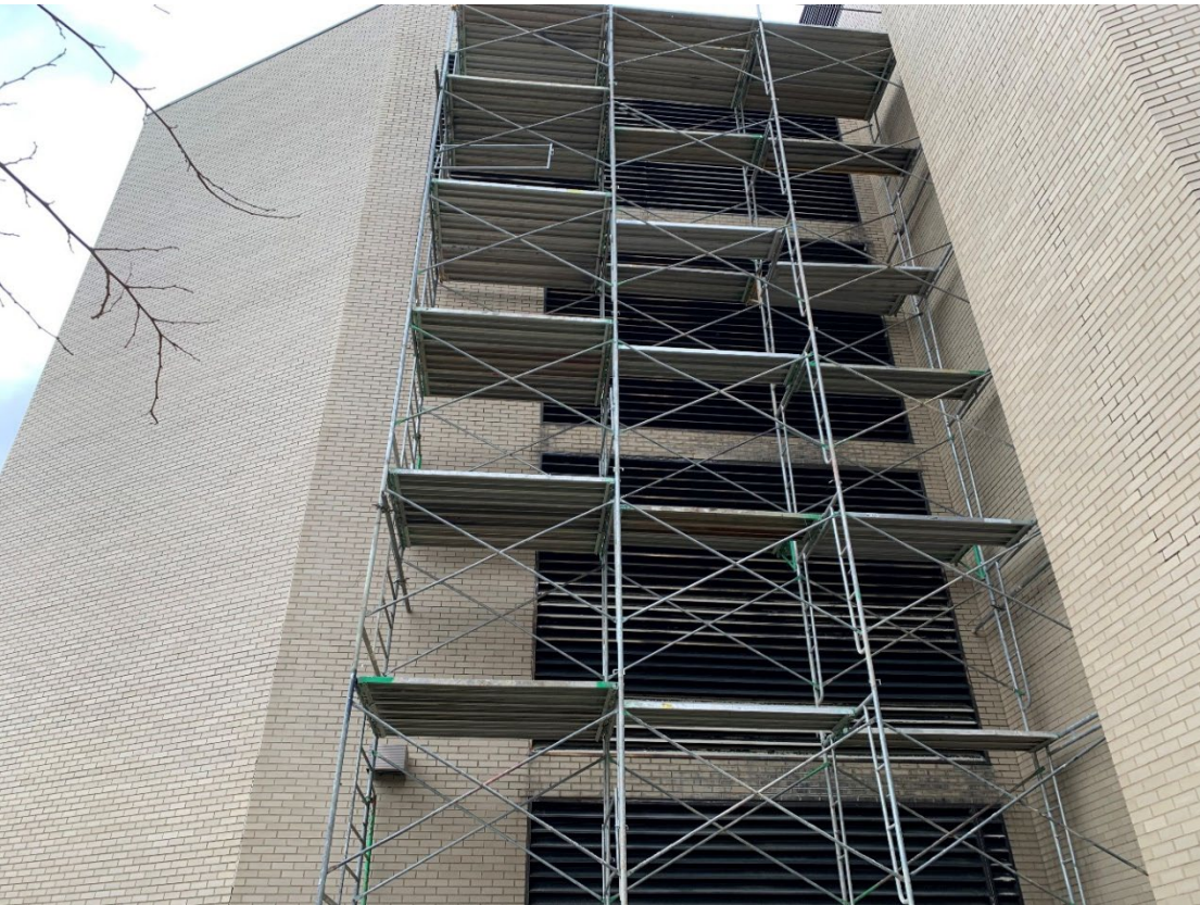
Campus Air Damper Replacements
