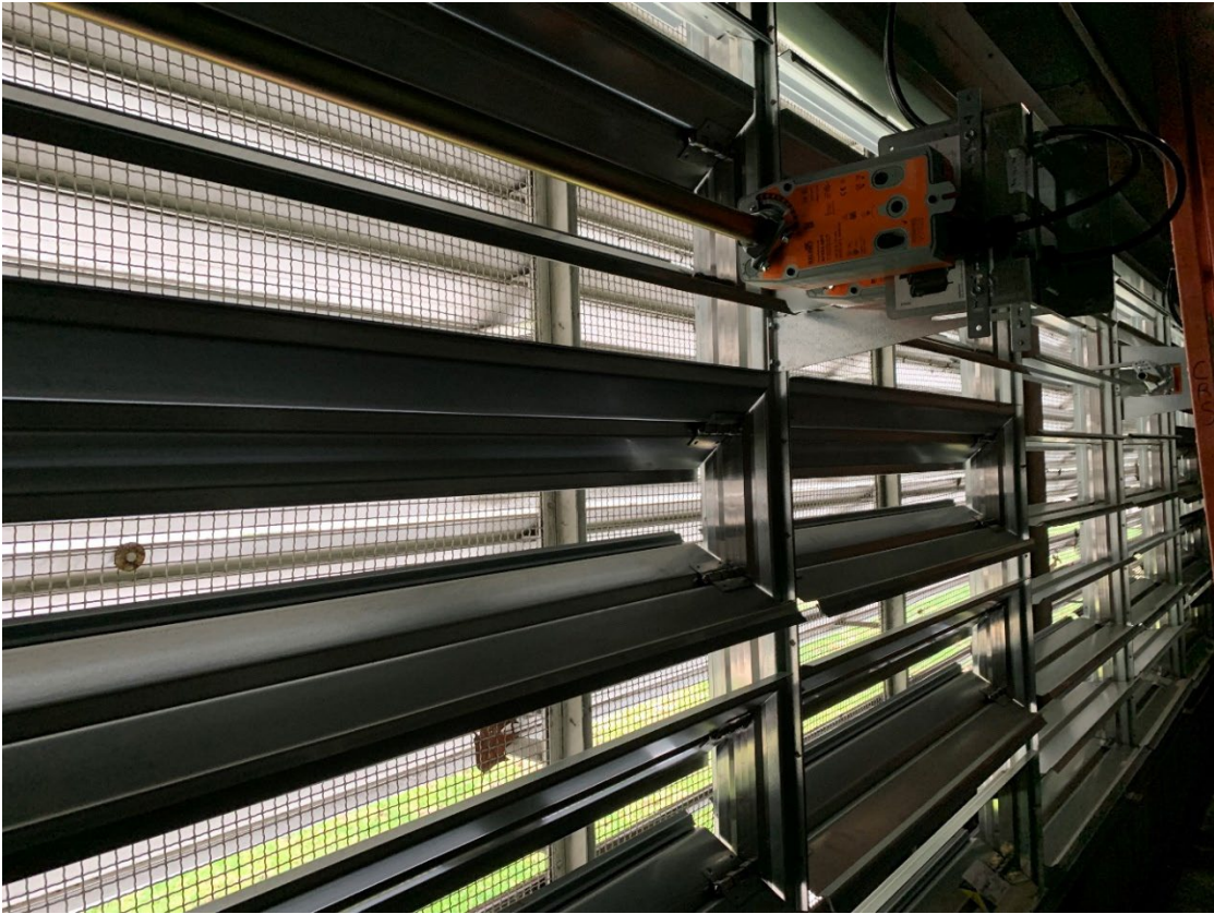
Campus Air Damper Replacements
